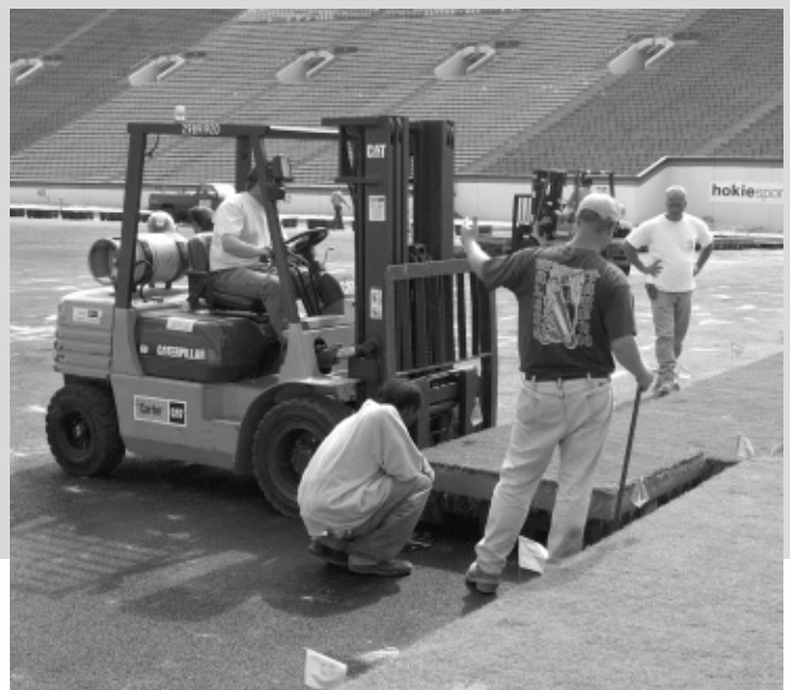
In July of 2001, workers installed the playing surface in trays on top of pavement that was laid down in Lane Stadium/Worsham Field.
