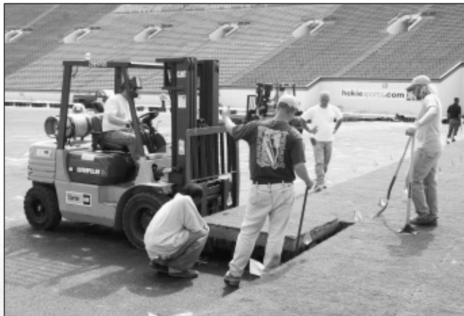
In July of 2001, workers install the playing surface in trays on top of pavement that was laid down in Lane Stadium/Worsham Field.
